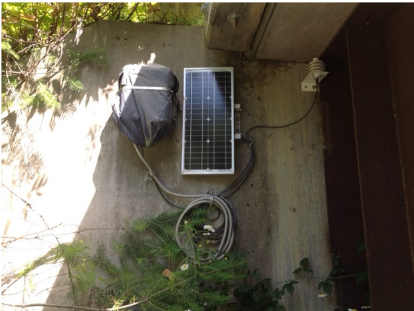
monitoring station fixed to left bank ballast wall
